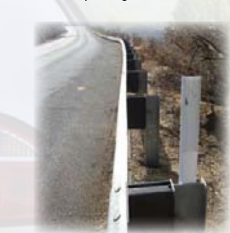
The new guardrail, along fire-prone areas of SR 94, features metal posts that can better withstand possible fires in the future.
